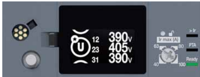
Voltages on panel display
